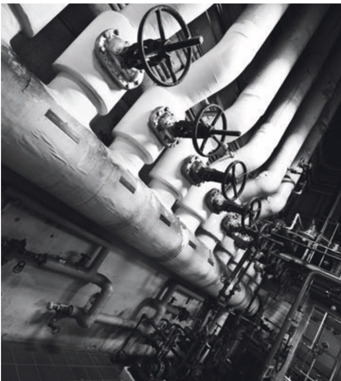
The boiler room, which is located in the basement of the Children's.
